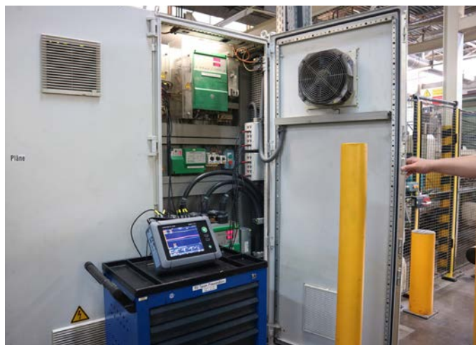
Acquisition of control signals from the PLC.
