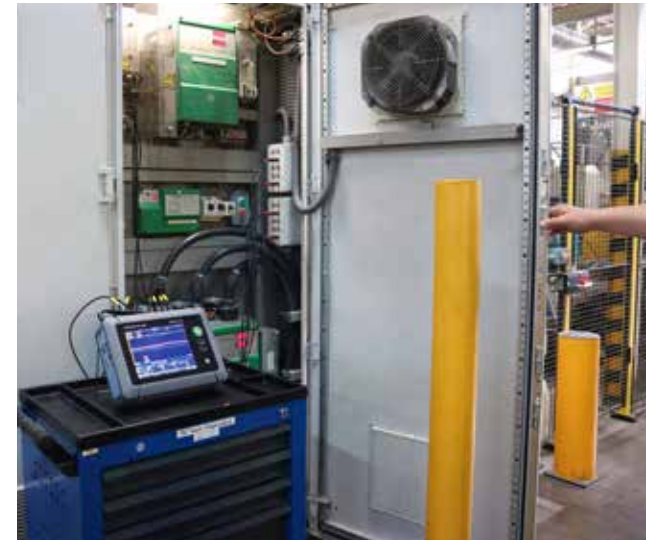
Acquisition of control signals from the PLC.
